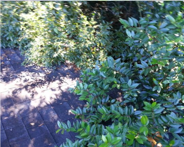
Tree contact on roof
