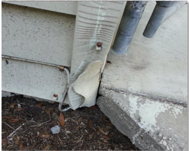
Miscellaneous damage to siding and trim
