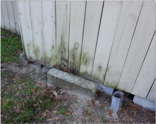
Deterioration to fencing
