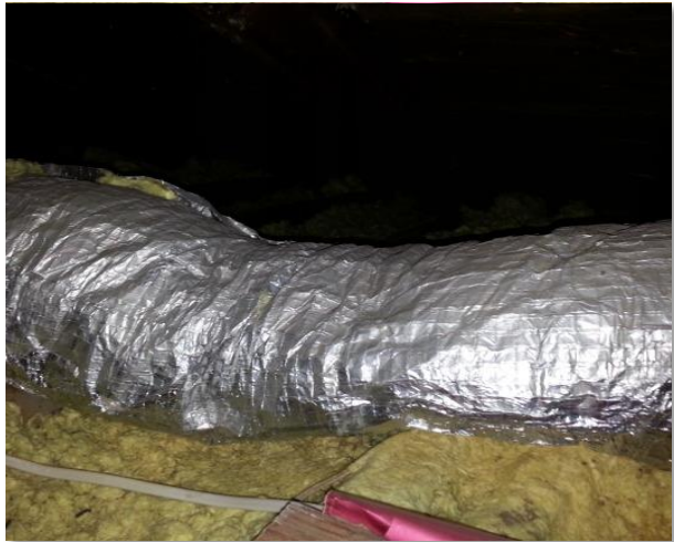
Example of deteriorated ducting in attic
