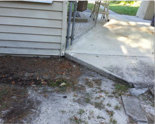
Erosion behind carport
