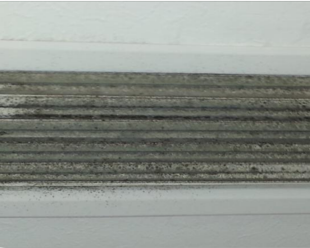
Example of mildew on AC registers
