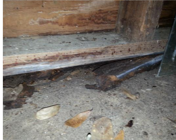
Rotted away bottom plate at garage wall framing
