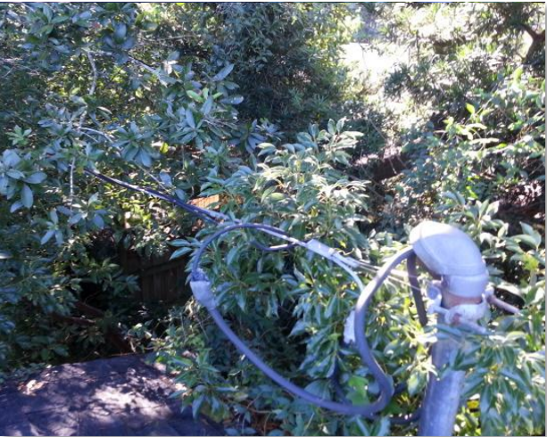
Main service wire going through trees
