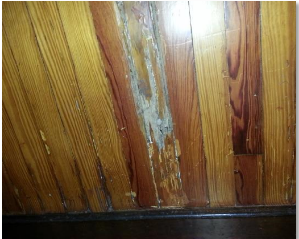
Badly damaged flooring in rear bedroom
