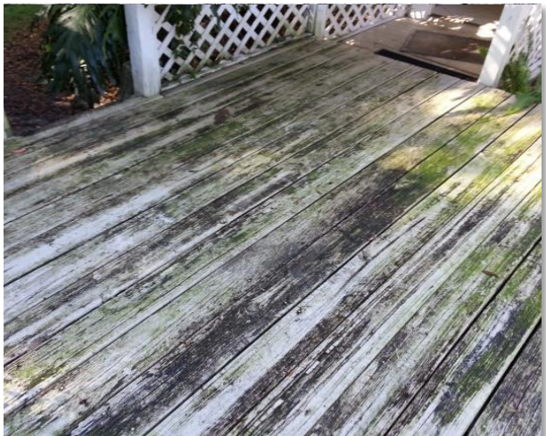
Deterioration to rear deck
