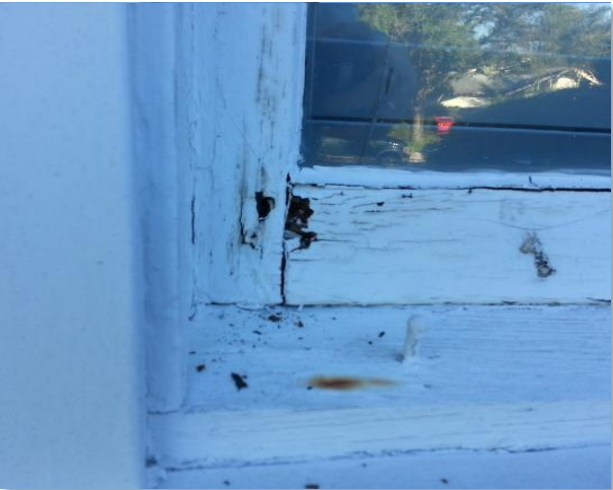
Decay at NW window
