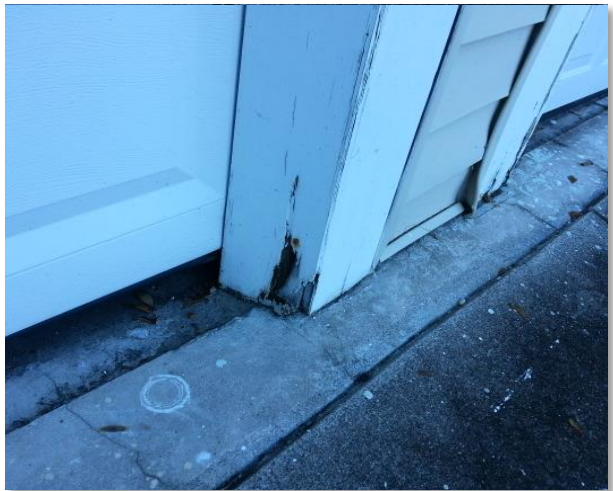
Decay to garage door trim
