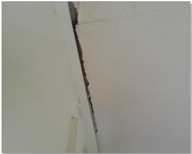
Settlement damage to plaster in apartment
