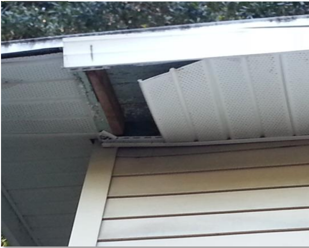
Loose soffit on west side of garage
