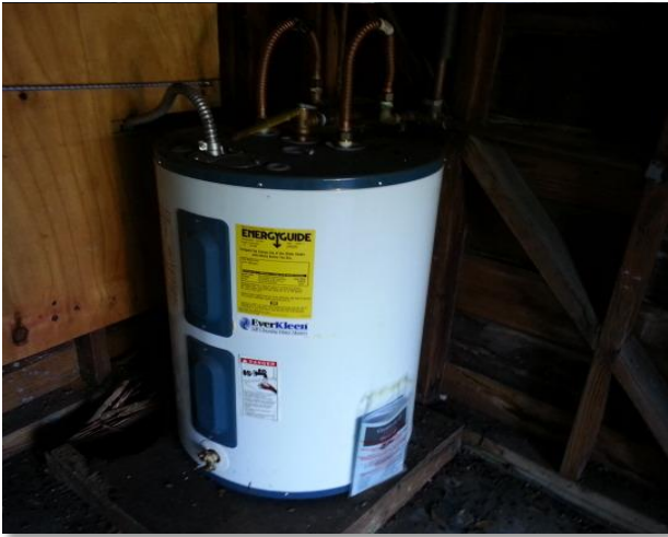
Apartment water heater
