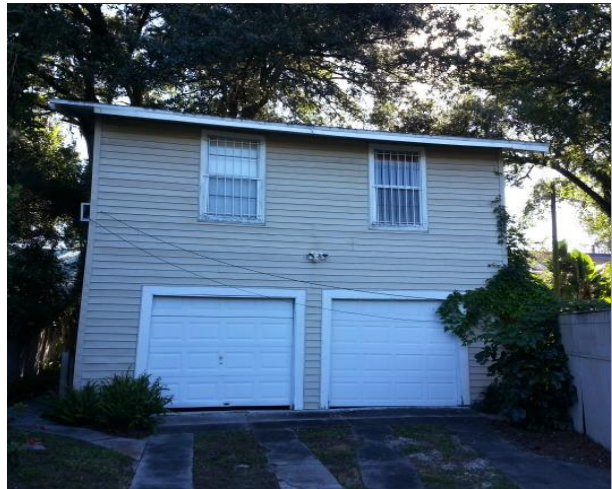
Garage view showing lean
