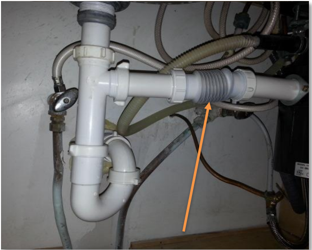
Corrugated piping under kitchen sink
