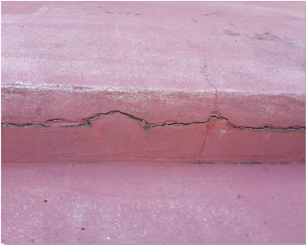
Cracking to front porch should be sealed soon
