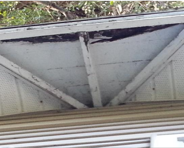
Rot and leakage at garage roof north edge
