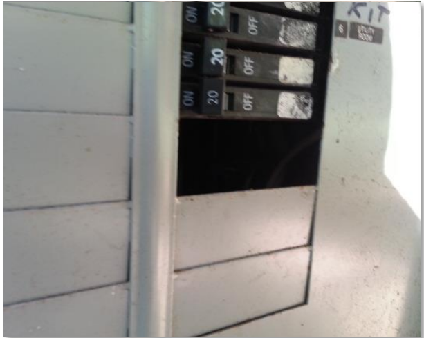
Missing knock-out at garage service panel
