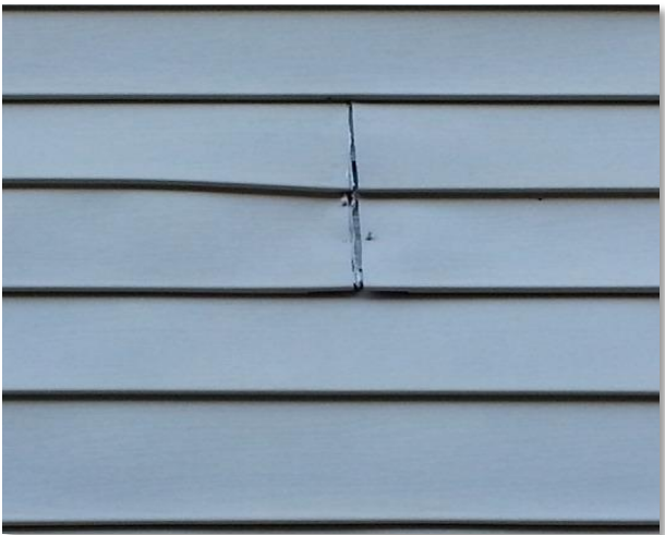
Split siding on upper front wall of garage
