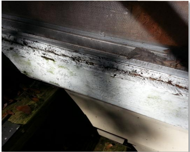
Rotted rear wall garage window sill
