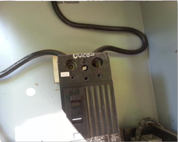
Over-sized breaker at garage service panel
