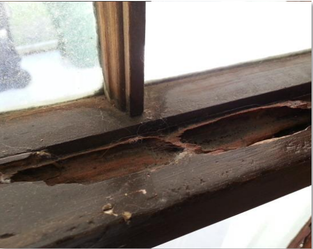
Example of termite damage to windows and other trim
