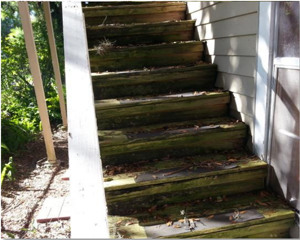
Garage stairs are very weak
