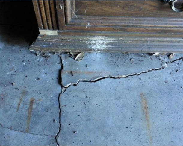
Cracking and settlement to the garage slab
