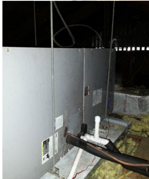
Air handler view
