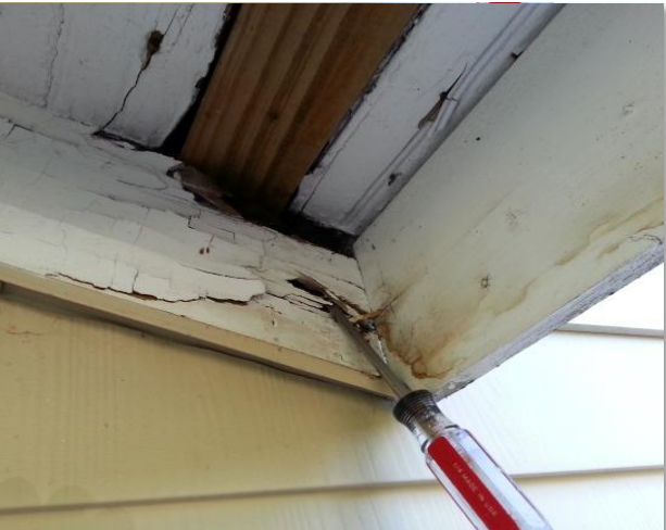
Decay at front entry roof rafter
