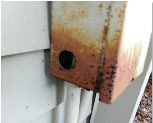
AC disconnect has missing knock-out and is badly rusted
