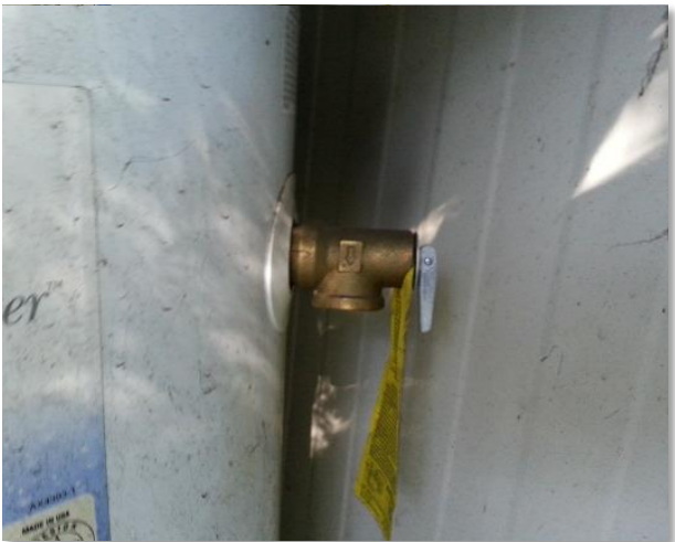
Missing TPR extension pipe
