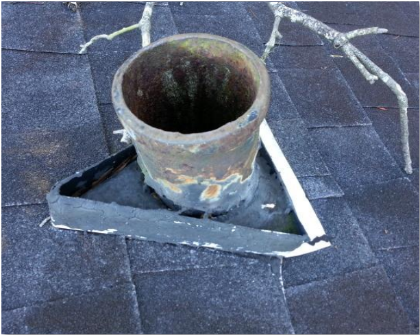
Improved sealant needed at pitch pans soon
