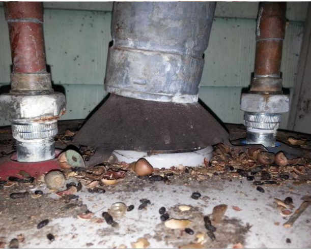
Improperly installed vent at main house water heater
