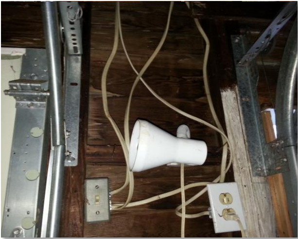
Many exposed wires in garage
