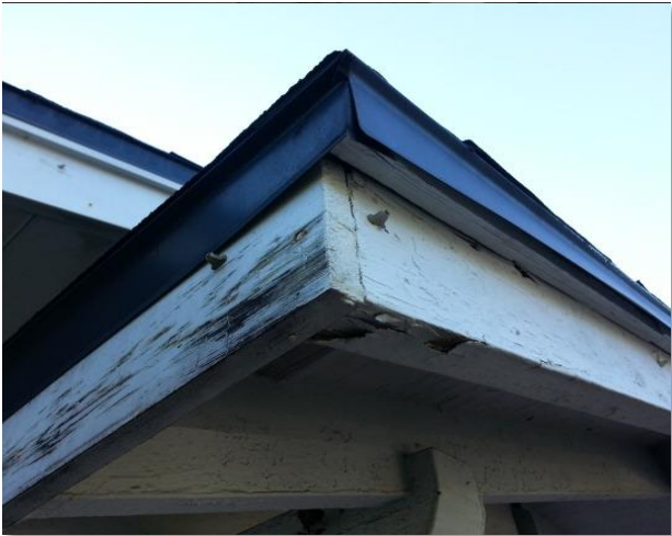
Deterioration to wood trim elements
