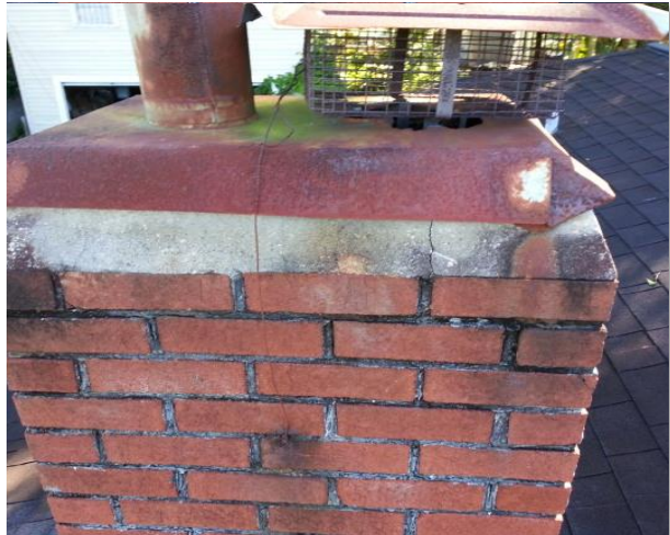
Deterioration to chimney
