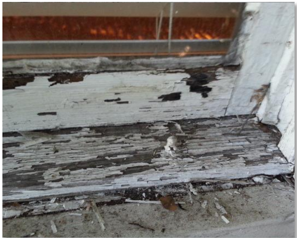
Rear bedroom window is badly deteriorated
