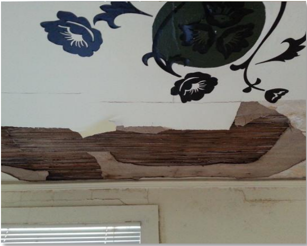
Water damage to plaster in apartment
