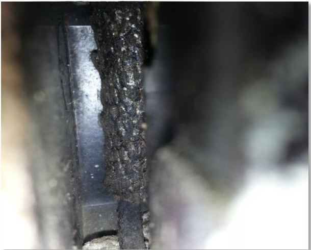
Knob and tube wiring seen in the apartment
