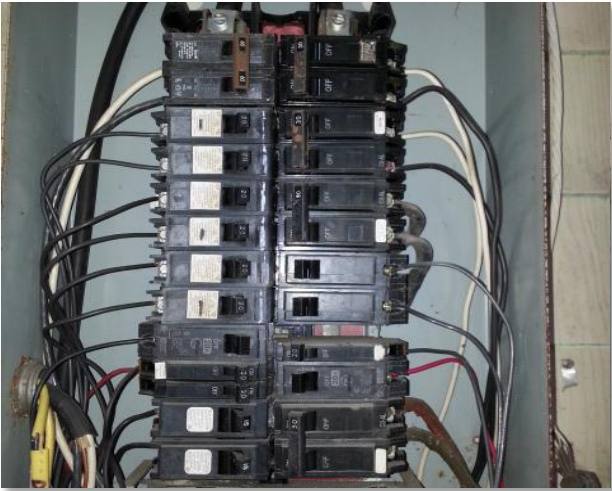
Main electrical panel
