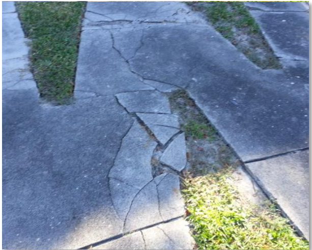
Damage to drive
